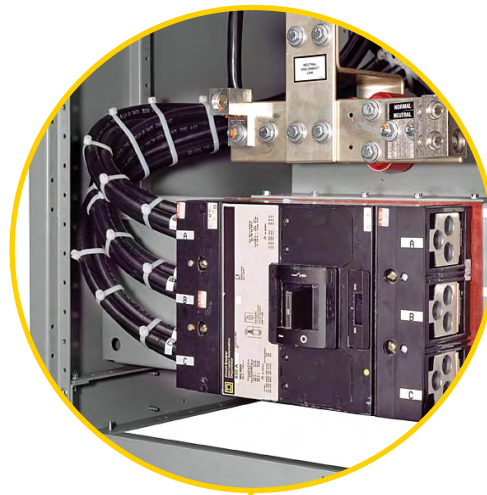
Service Entrance Breaker
